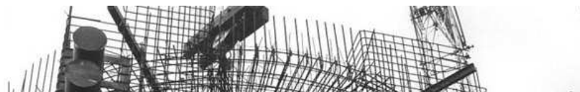
Installation of reinforced shell for the first reactor of Zaporizhia NPP to be filled with concrete, 1982. Photo from seogan.ru
