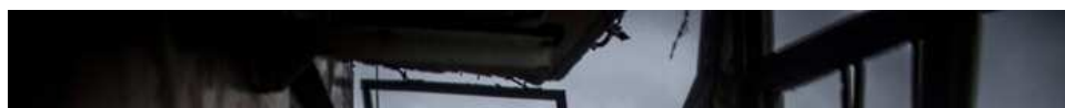
A broken balcony in a residential building damaged by mortar fire of Ukrainian forces in Lugansk. (RIA Novosti / Valeriy Melnikov)
